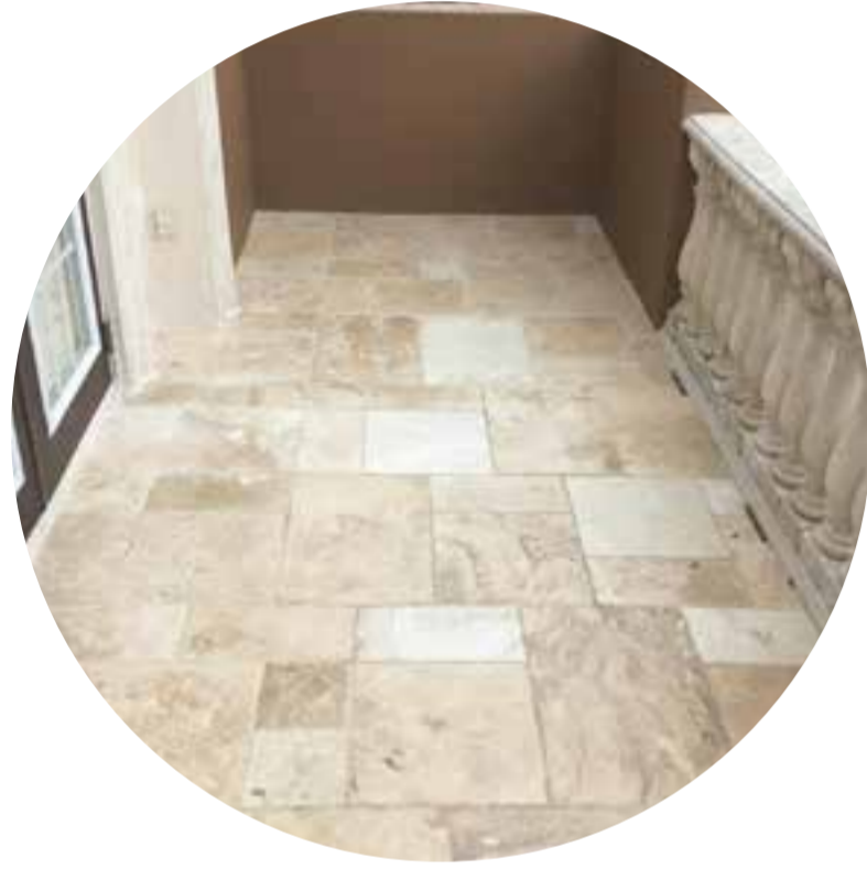
2. DECK WITH TILE, PAVERS OR TRAVERTINE VFI-600 Series Acrylic Roofing System with VFI-608 Below Grade Waterproofing
